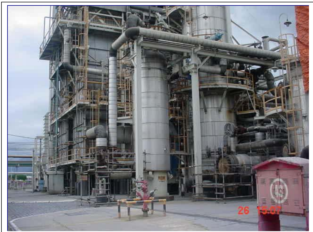
This picture shows the new installed pre-reformer
