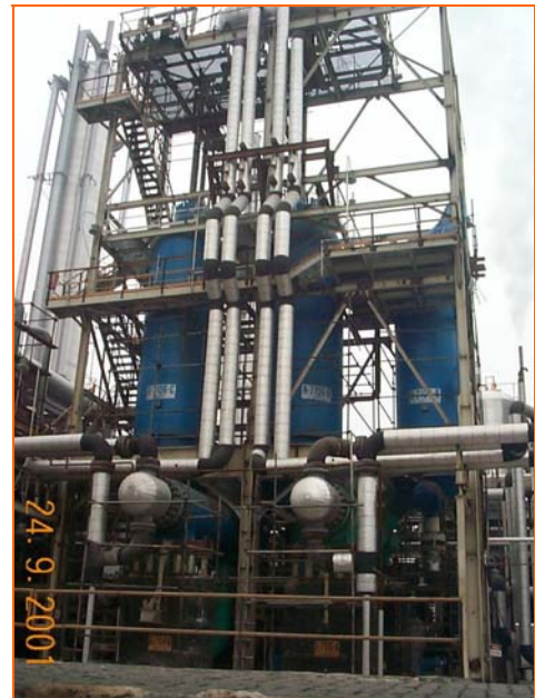
This photograph shows the three new converters and the HP waste heat boilers
