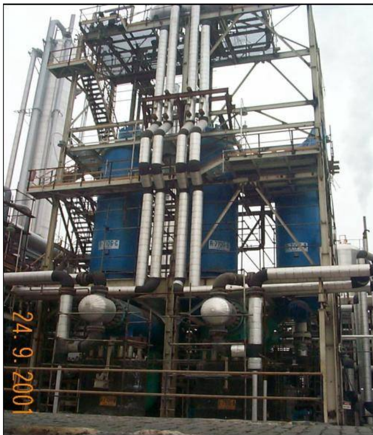
Fig. 5: The three new converters and the HP waste heat boilers
