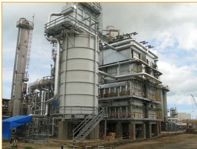
Fig. 8 – Photo of the Primary Reformer and Fired Heater
