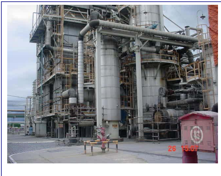
Fig. 4: The Recently installed Pre-Reformer
