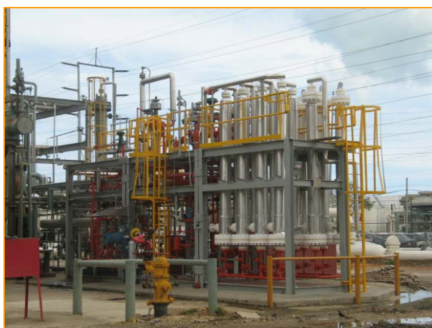
Fig. 9 - Photo of the Refurbished HRU
