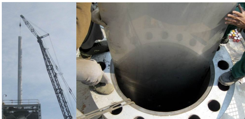
Picture 2: Converter modules insertion in the vessel
