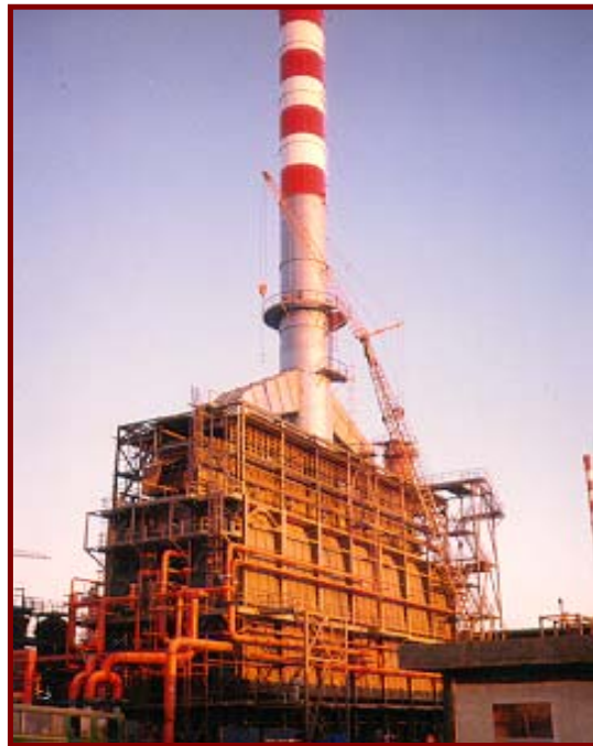
Terrace Wall Steam Reformer - 50,000 Nm 3 /h Hydrogen plant
